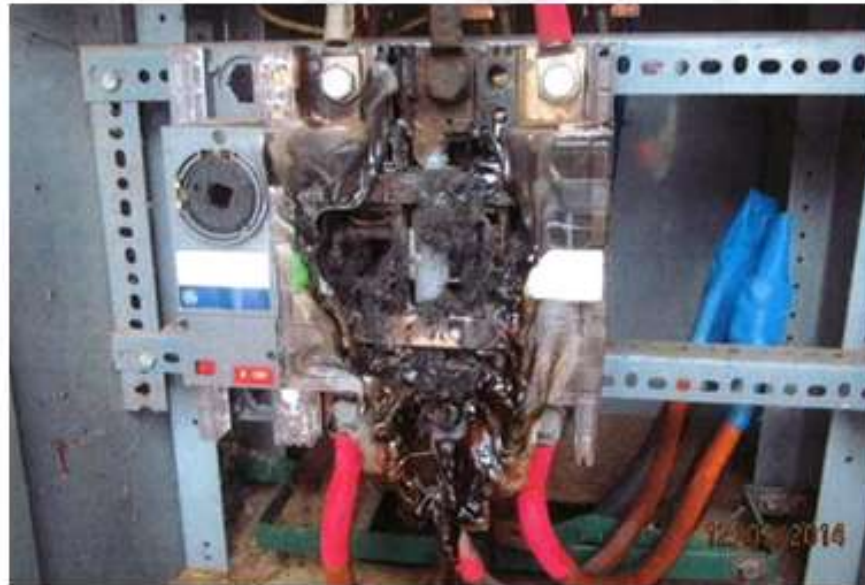
Photograph of the main isolating switch at Otonga Pumping Station
