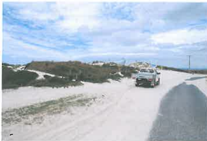
The race course vehicle entrance showing what the regular inundation looks like (2m+)
